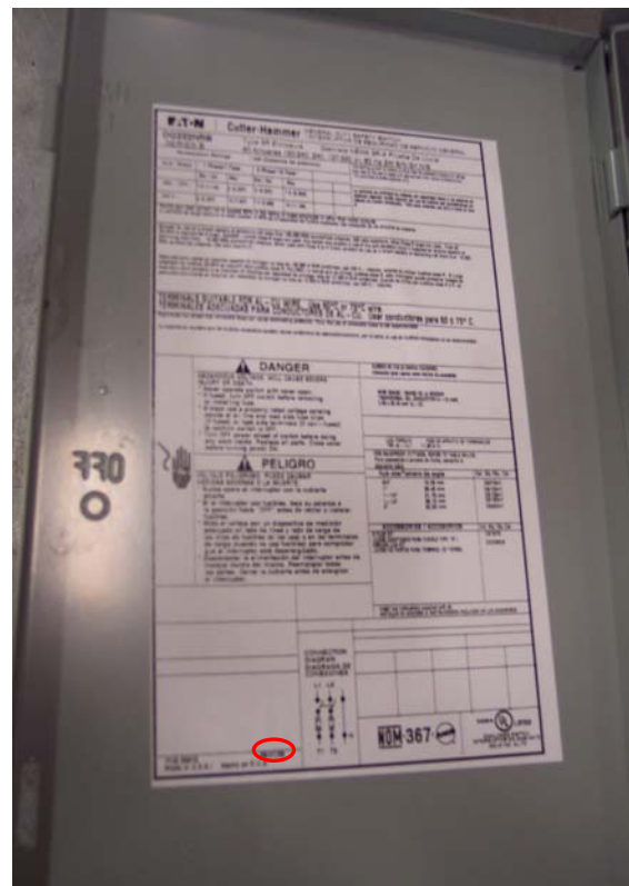
Figure 3. The red circle indicates where the date code is located on the pub inside the case of the switch
